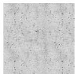
MASONRY CONCRETE SPLINTERED
