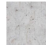
MASONRY CONCRETE STAINED
